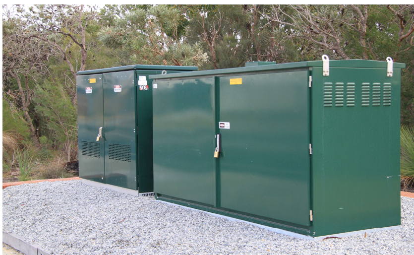
Figure 57: HV outdoor ground mounted switchgear & transformer
