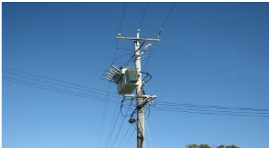
Figure 58: HV outdoor aerial mounted equipment
