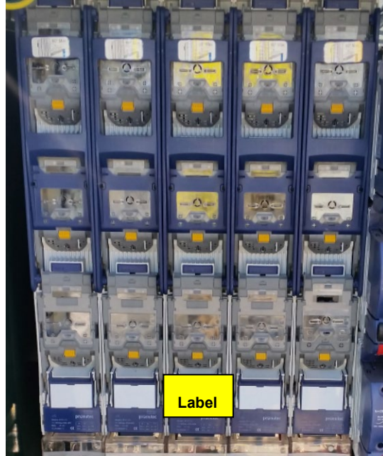
Figure 27 – ‘Pronutec’ Fuse Switch label location.
