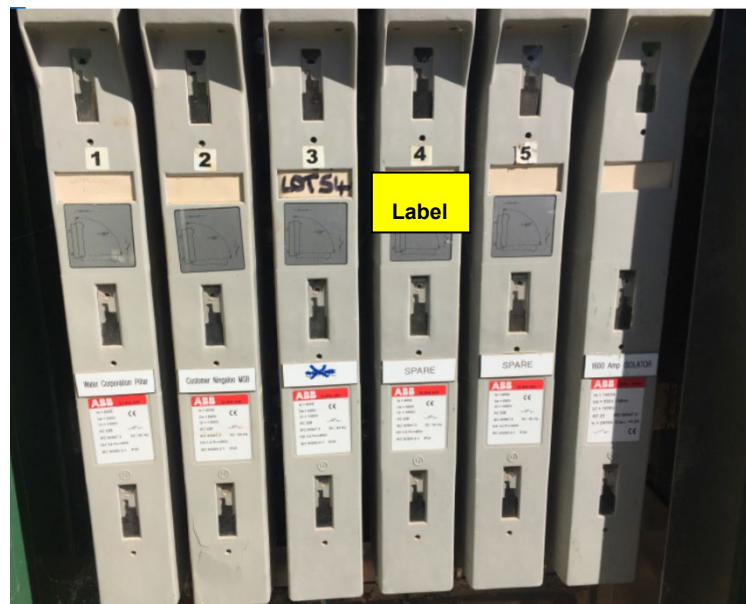
Figure 28 – ‘ABB’ Fuse Switch label location.
