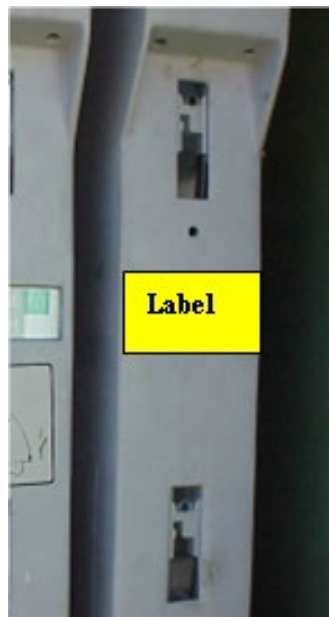
Figure 23 – ‘ABB’ LV Disconnecter label location.
